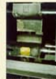
GAUGE MOUNTED TO OTHER EQUIPMENT
